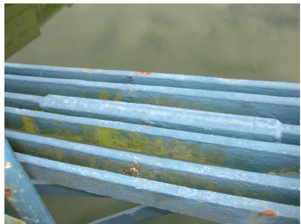
Figure 14: Algae, rust and repair to damaged link
