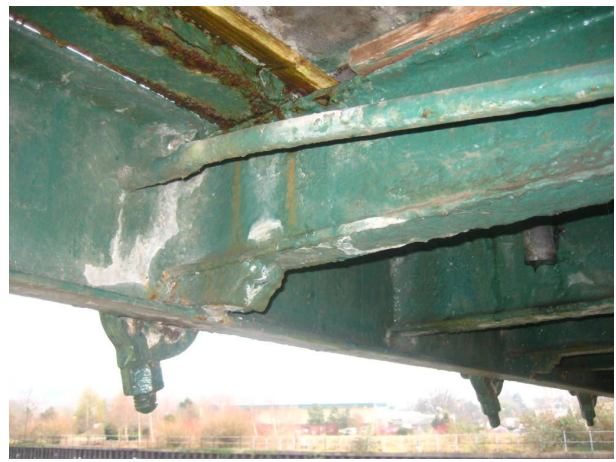
Figure 13: Corrosion to the underside of the deck above towpath.
