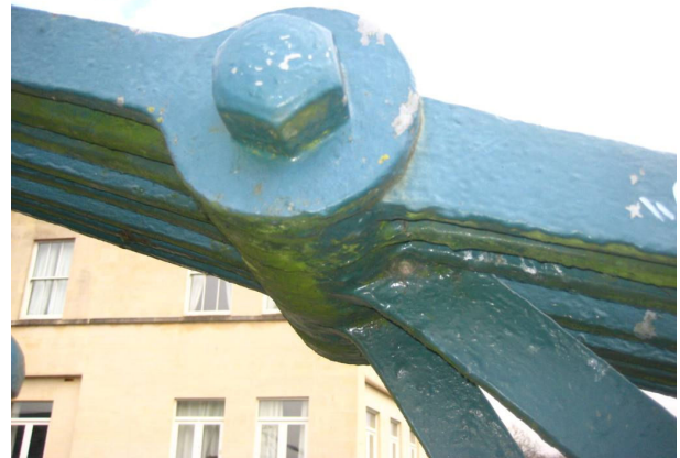
Figure 3: Bolted connection on the chain, note that the number of links reduces from 8 to 7 at this node
