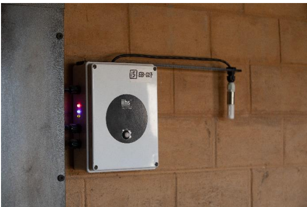
Figure 2 An IoT Box installed at a room level
