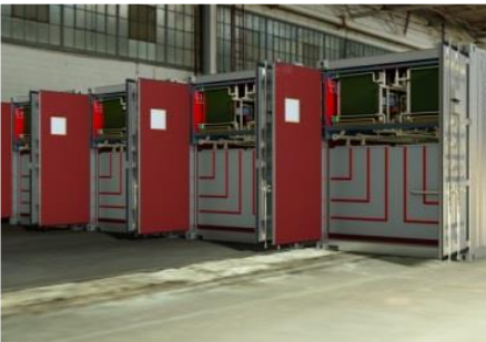
Grid scale Flow Battery
