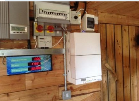
Lithium ion domestic battery
