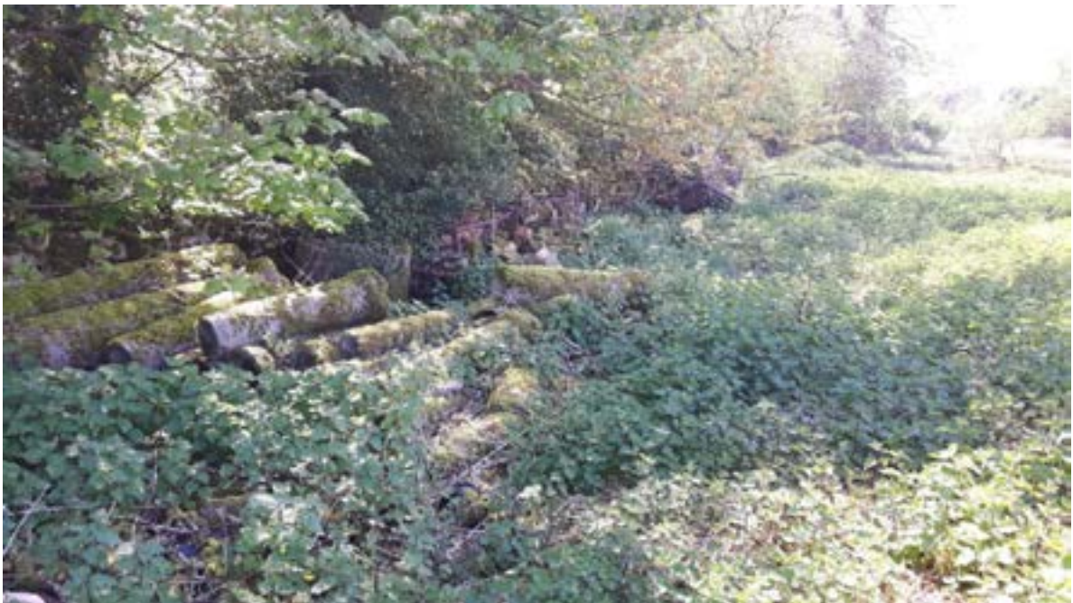
Plate 10: Possible asbestos pipes (as identified as T1 on Figure 1)
